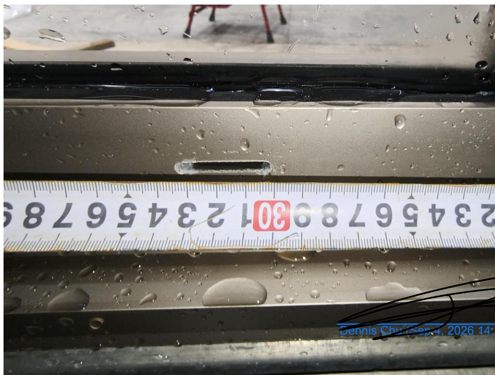
Figure 10 Photo of Drain Holes Detail
