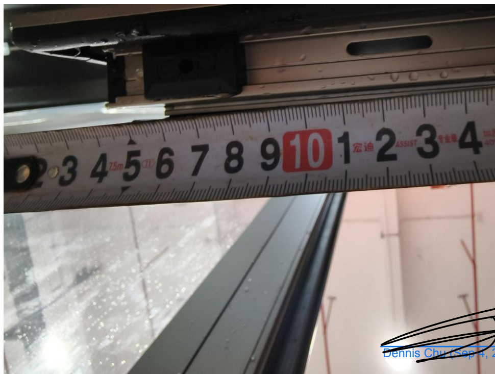
Figure 11 Photo of Drain Holes Detail
