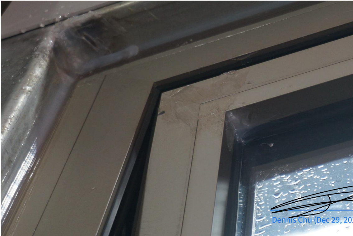
Figure 19 Connection Detail of Left Side Jamb, Head Jamb, and Operable Sash (Opened Position)
