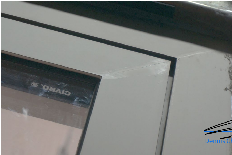
Figure 18 Photo of Top Right Corner of Door Frame, Top Rail and Stile (View from Exterior) (Showing White Traces Left by Transparent Waterproof Coating on Surface)
